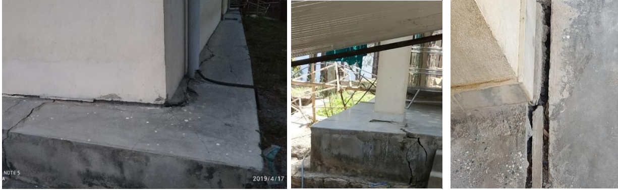
Figure 6: Cracks and settlement CEONC building walls and apron
