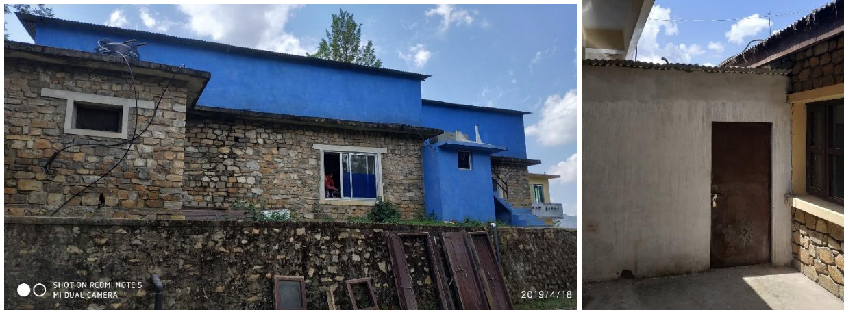
Figure 9 Extension of floor on the delivery block and biomedical engineering department (left) and additional blocks (right)
