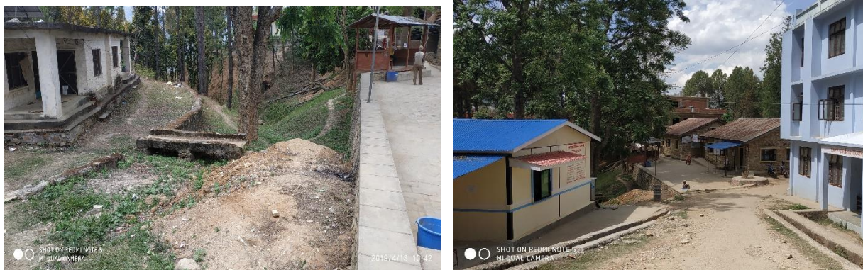
Figure 12: Drainage channel with C&D waste (left) and access road and drainage in front of hospital compound (right)
