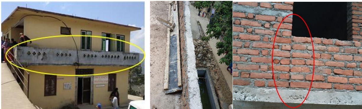
Figure 8: Vulnerable parapet (left) and inadequate brick bonding (right)
